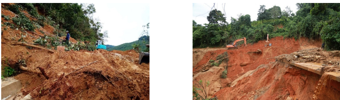
Figure 2 Landslide along roads in Quang Nam province
