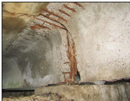
Figure 1– Corrosive destruction and degradation of cement concrete with exposure and corrosion of reinforcement of the bridge over the Svyatukha River at km 48+718 of the A-215 highway.
